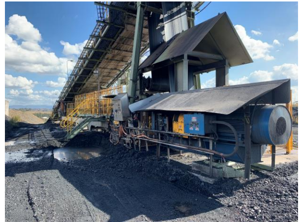
Figure 2. Main Conveyor Drive Head
