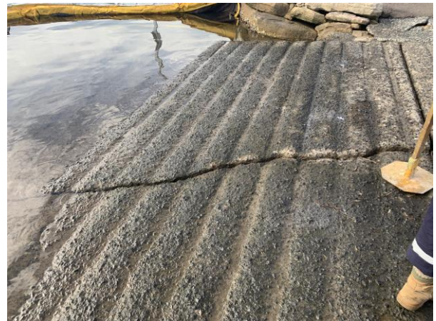
Figure 2: A concrete slab close to the water which showed signs of subsidence
