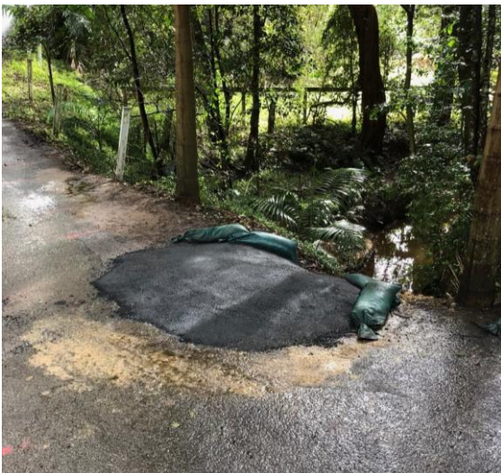
Figure 3: The consolidated sinkhole with the applied bitumen
