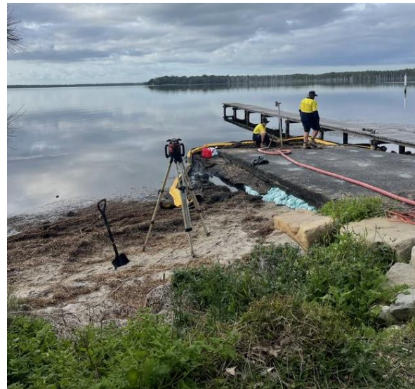
Figure 2. The Resinject team working to fill the voids beneath the boat ramp
